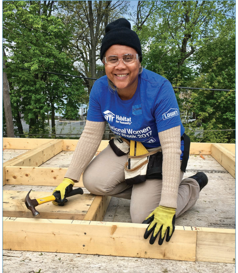
Elisemene Volmar is hard at work doing her sweat equity. Like all Habitat homeowners, the Volmar family put in 300 hours on the construction site.
